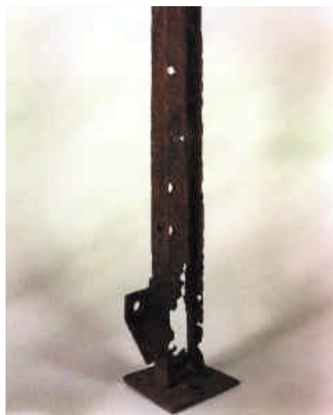
Figure 11 Corroded steel stanchion
