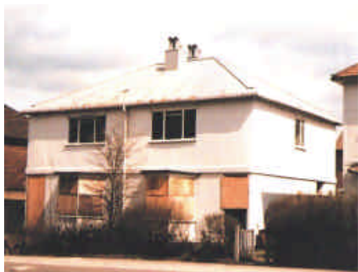
Figure 1 Telford steel framed house -1920s - this was one of the steel clad systems
